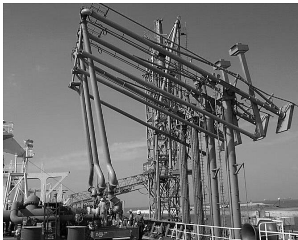
Fig. 1. Loading arms for loading/unloading tankers in the oil terminal [6]
